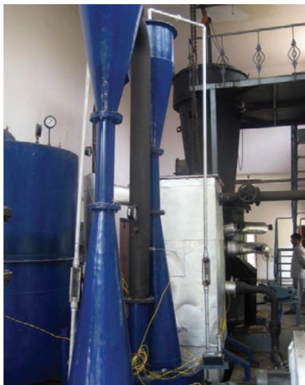
The biomass-gasifier uses a gas engine to produce electricity; waste heat from the engine runs the desiccant refrigeration system. CSIRO
